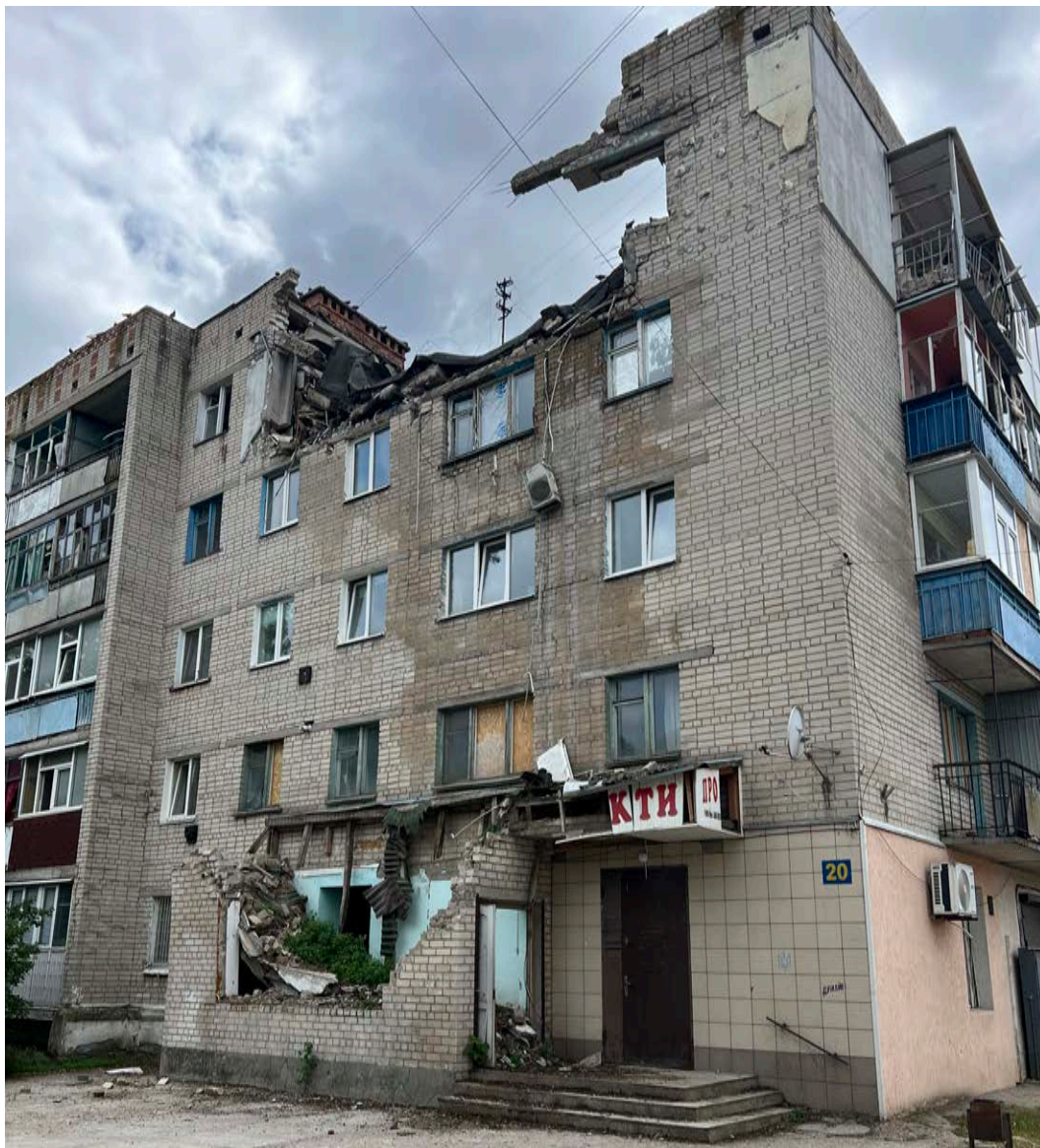
Elena's building in Kivsharivka badly damaged by missiles.
