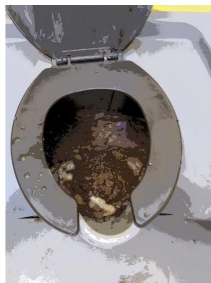
Figure 45 an overflowing latrine in the camp. Currently the camp has roughly half the recommended number of latrines forcing many residents to utilize the woods or the river.
